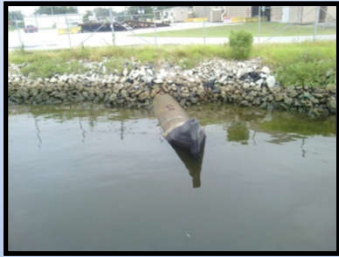
Exterior Check Valve
