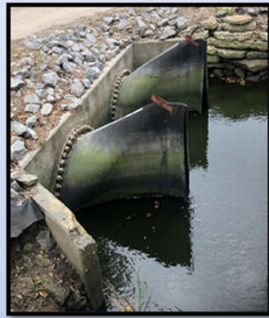
Exterior Tideflex Valve Howe Street Outfall
